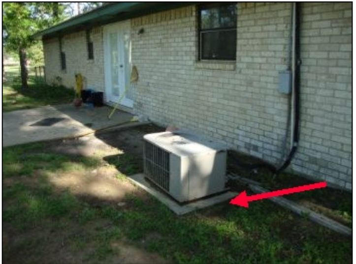
A/C unit should be made level
