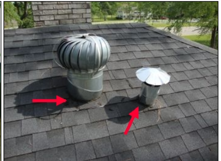
Flashing not reset when roof was replaced
