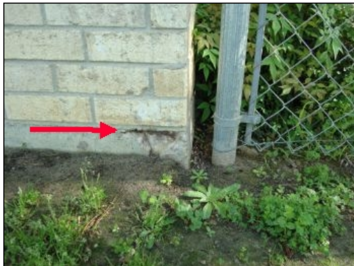
Corner of southeast slab has air pocket
