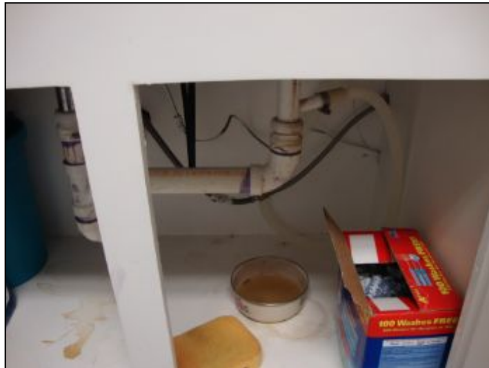
Leak found under kitchen sink
