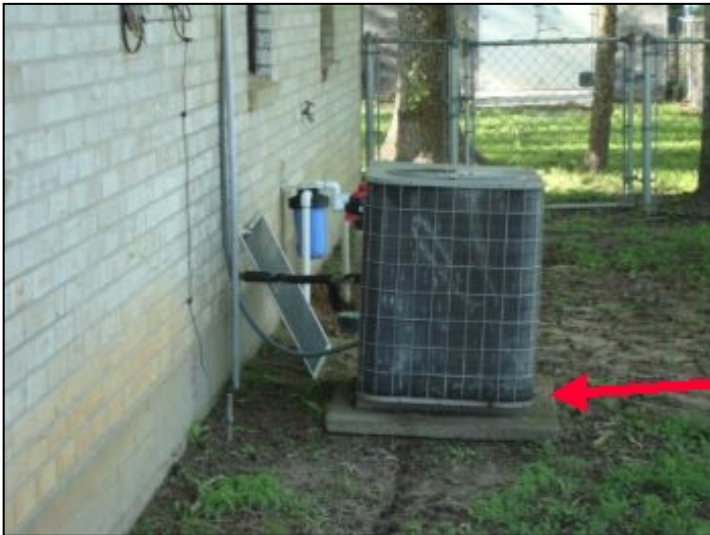
A/C unit should be made level
