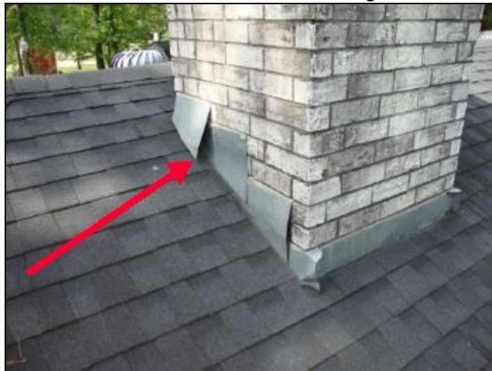
Counter flashing pulling away from chimney
