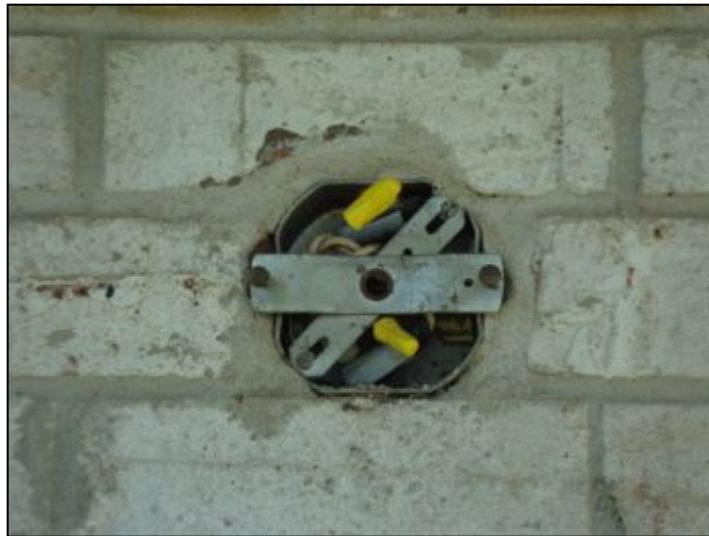
Missing light fixture and exposed wires
