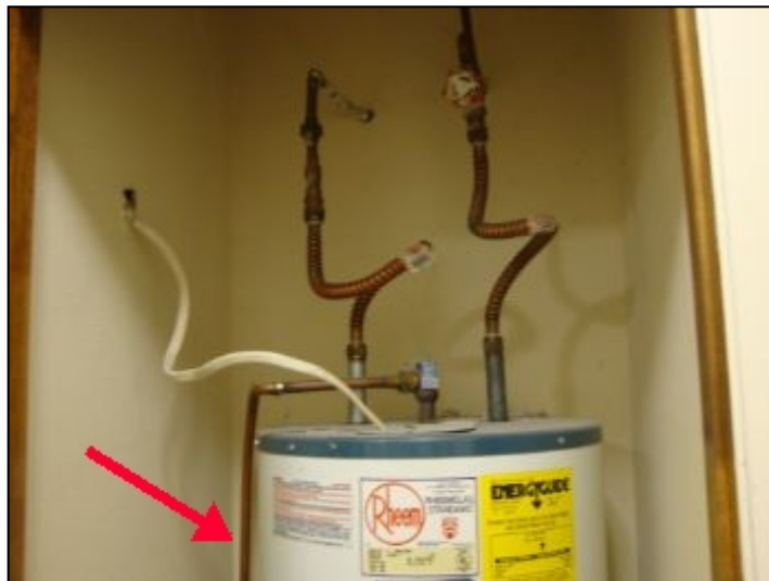
No drain pan and T&P relief valve drain pipe is installed improperly
