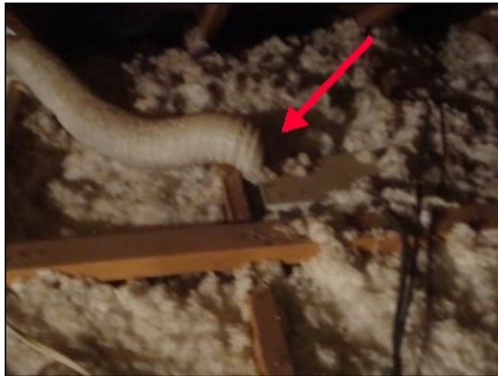
Bathroom vent fan exhaust tubing pinched
